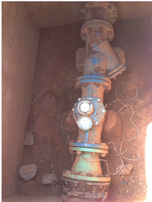
Figure 2–3: Bulk Meter for A1 (SSNIT)
