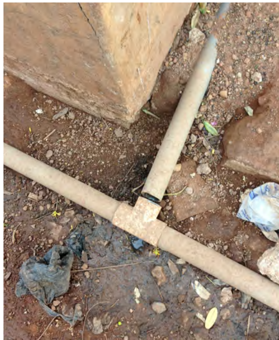
Figure 6–2: Broken pipe in Old Cemetery neighborhood (indicating a possible route of contamination)
